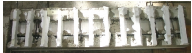
Figure 23. Flat-panel ICF lintel with low slump concrete vibrated with an orbital sander. (IMG13355)
