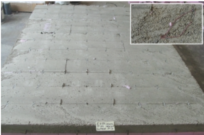
Figure 29. Full height flat-panel ICF with medium-high slump concrete (no mechanical vibration). Note the closeup view of an area with segregation. (IMG13379, IMG13624 [insert])
