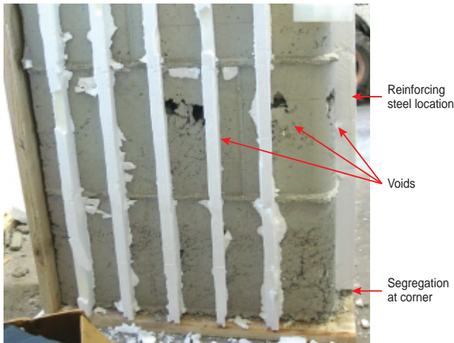
Figure 20. Flat-panel ICF corner configuration with medium-high slump concrete (no mechanical vibration). (IMG13352)
